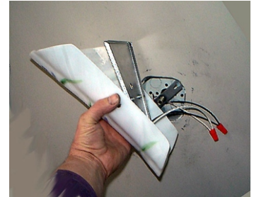
Sconce with wires attached to wall supply by wire nuts.
